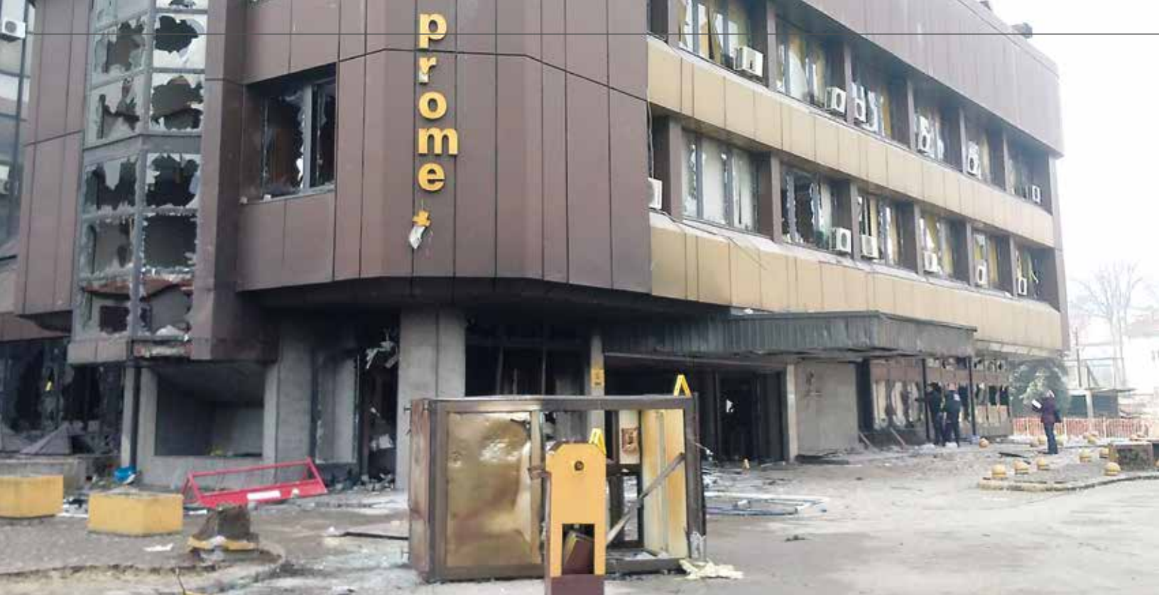
Zenica-Doboj Canton building the day after the riot in February 2014
