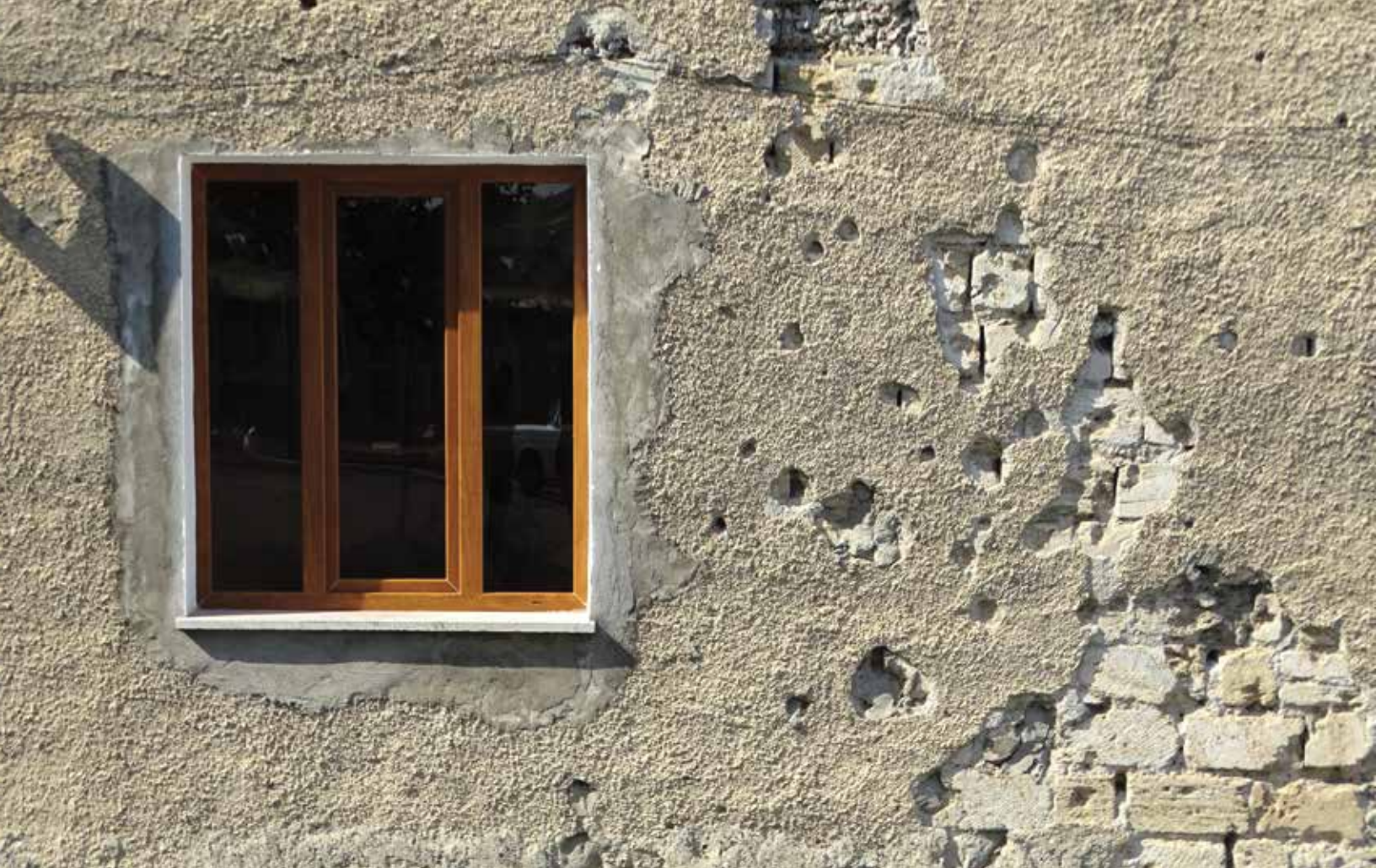
Shell-pocked facade, Stepanakert, Nagorno-Karabakh. Photo by Adam Jones (2015).
