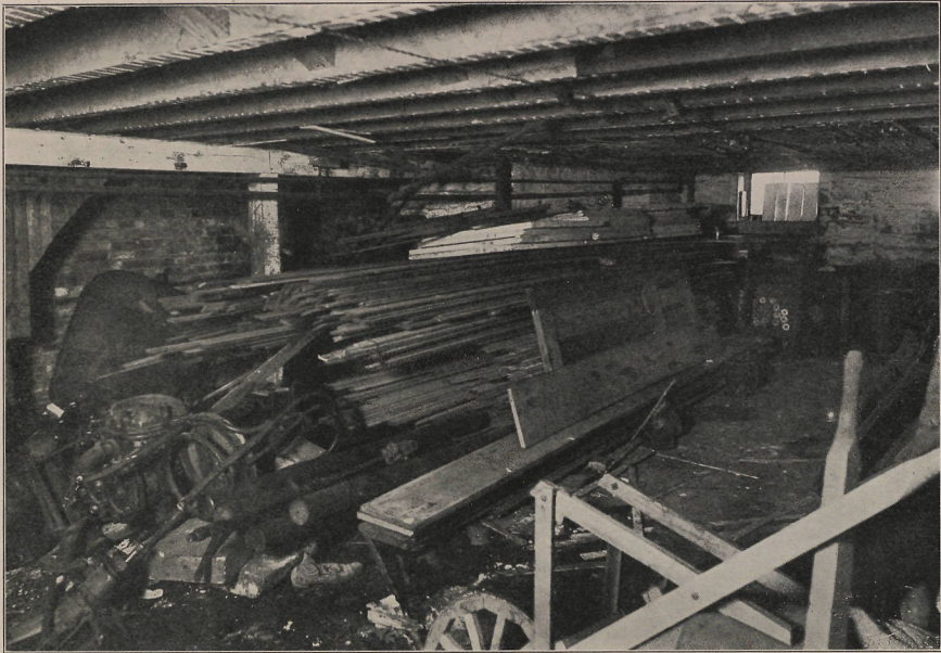
PHOTO. 16.—AN INVESTIGATION BY THE BUREAU OF SUPPLIES DISCLOSED THIS CONDITION. (Valuable stock stored with junk in the cellar of a pumping station.)
