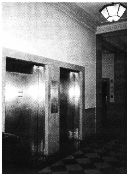
All three passenger elevators have been completely replaced in Phase 3 of the renovation. New machinery results in faster moving, more efficient elevators. Stack elevators will be renovated in a future construction phase.
