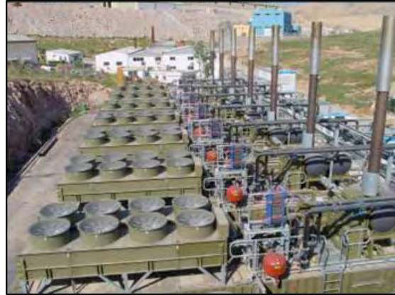
Figure 4.59 Mobile energy production modules (50) .
