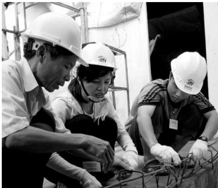
Volunteers bind steel for a Habitat house in My Tho, on the Mekong Delta.
